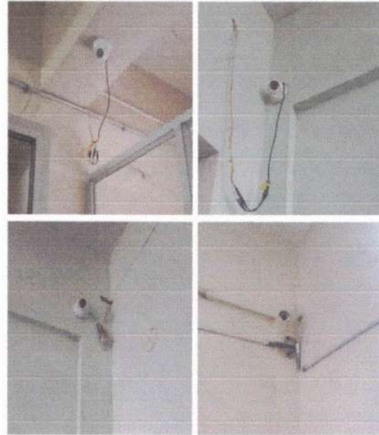
CC Camera Survivance at classrooms
